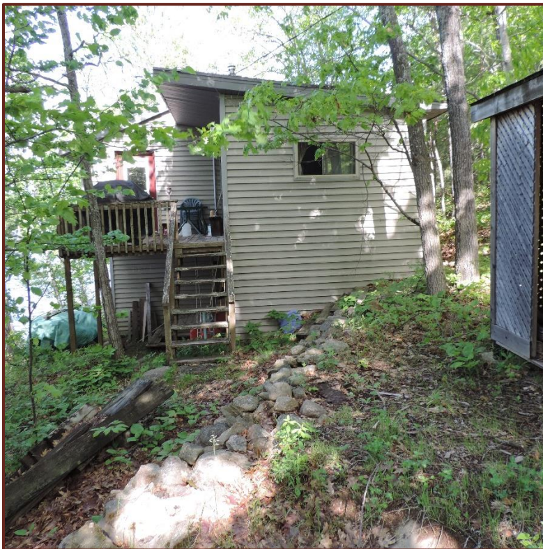
Photo 2. View of the existing conditions in the area where the deck extension is proposed.
