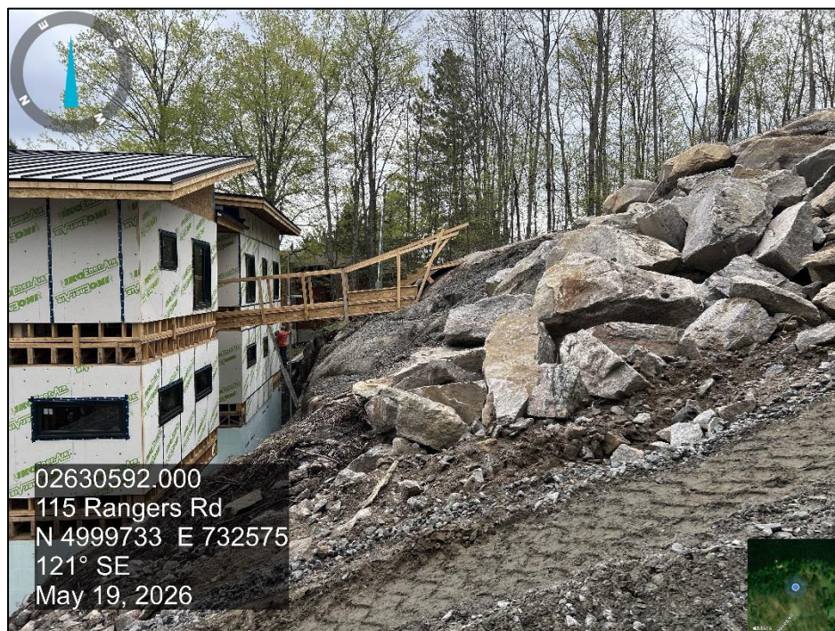
Photo 5 View of the top of slope near the slope face, looking east, showing the residential structure under construction, exposed bedrock, and loose boulders along the top of the slope.
